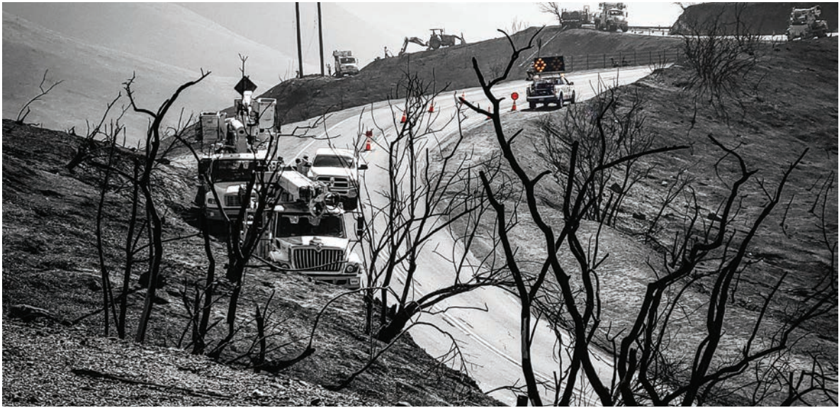
With scorched earth all around from the Woolsey Fire, Traffic Management Inc. maintains a road closure so that utility companies can repair and replace power poles.
