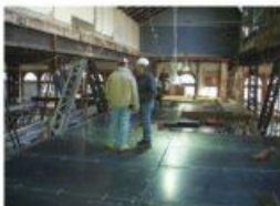
The flooring is a structural composite with two metal plates bonded by a polyurethane elastomer core.
